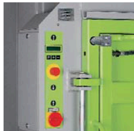
The control panel
