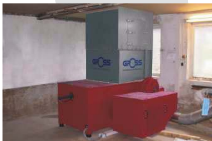
GAZ 102 set up below ground, with hopper expansion
