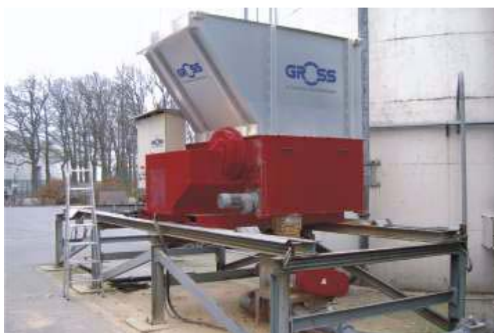
GAZ 122 on mount with extraction
