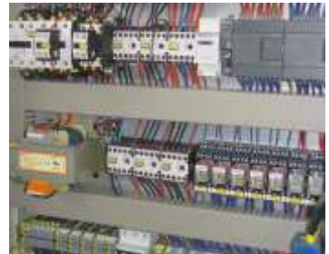
Switching cabinet / SPS control
