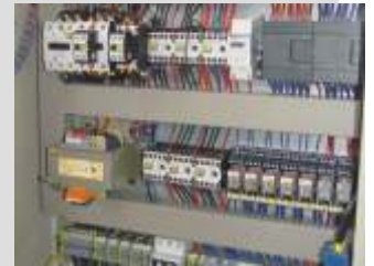
Control cabinet / PLC controller
